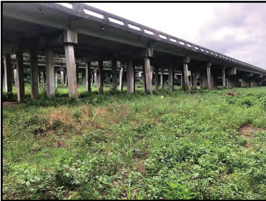
Portion of the Wateree River bridge through the floodplain, east of the river.
