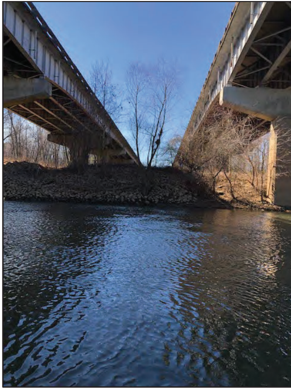
Plate 5. View of the Western Shoreline with rip-rap rocks between the I-20 Bridges. Photographer: Ralph Wilbanks; Date: February 01, 2022)
